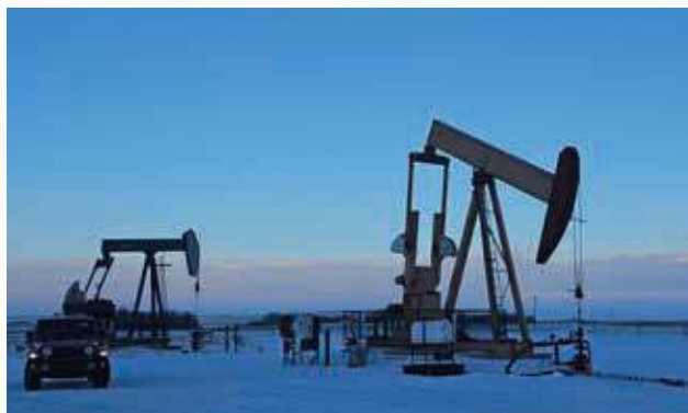
Pumping unit of well pad
